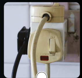
Overloaded sockets and extension leads.
